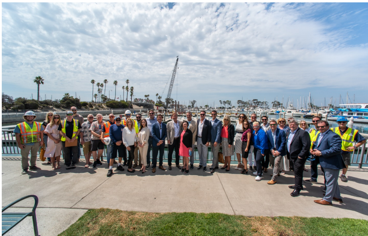
Joe Ueberroth and his partners, Scott Burnham and Bryon Ward are joined by Supervisor Lisa Bartlett and Mayor Joe Muller along with County, City and OC Parks staff for the pulling of the first pile, commencing the start of the marina’s construction.
