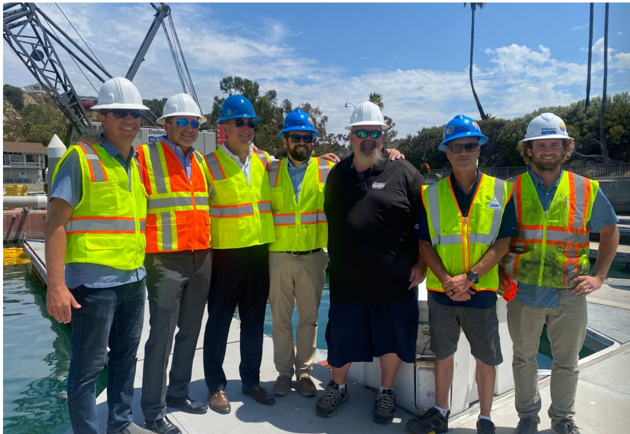
Joe Ueberroth is joined by fellow Bellingham team members after the pulling of the first pile.
